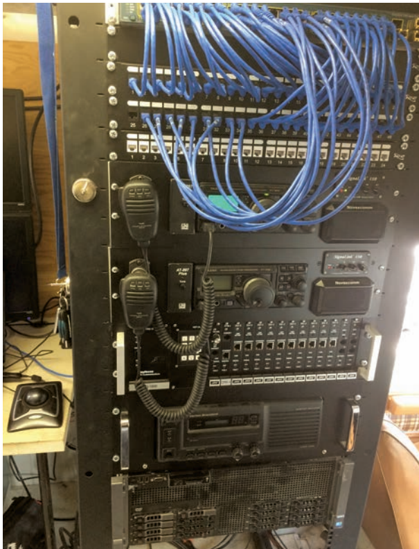
FIGURE 10. Servers, VHF radios, and switches are rack-mounted behind the driver's seat. Operator stations are to the left, and the radios can be operated from the driver's seat as well.
